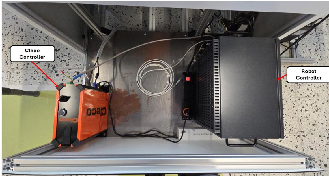
Figure 2: Interior view of the robot cell cabinet
